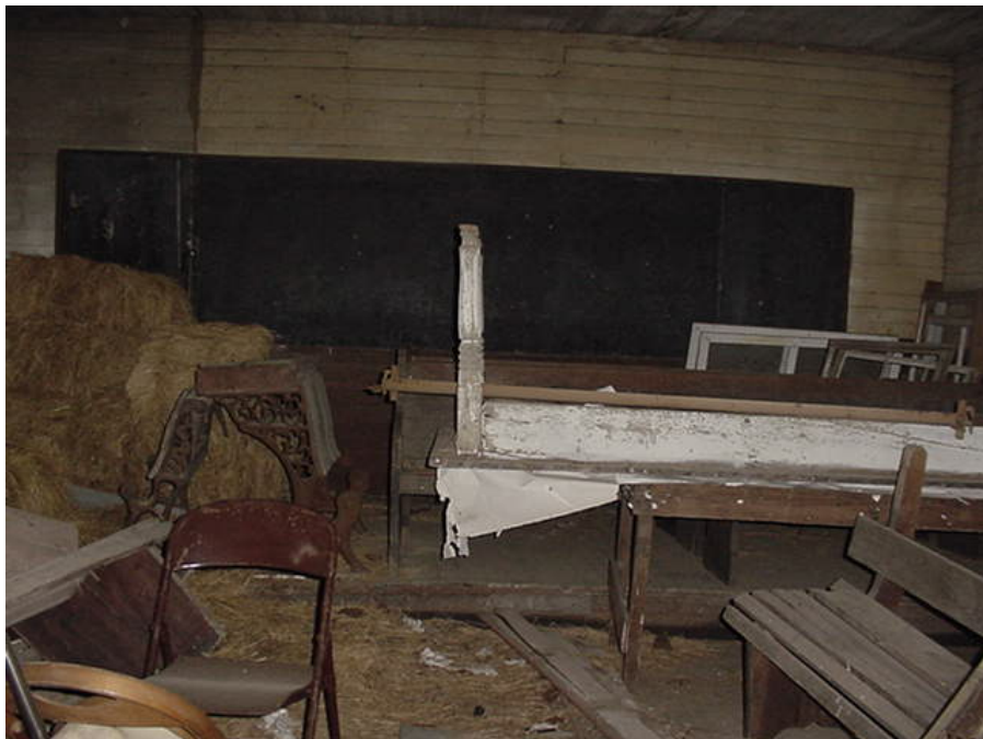
B10. Saunders Chapel School, Interior: Blackboard, Platform, And Current State of Disrepair
