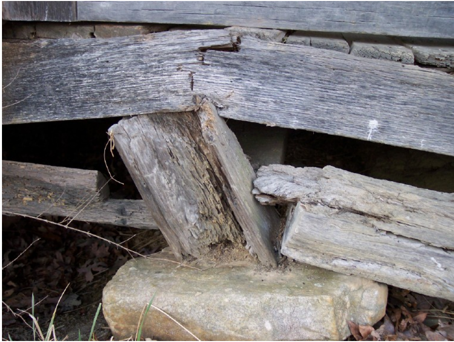
B5. Structural Damage to Floor System
