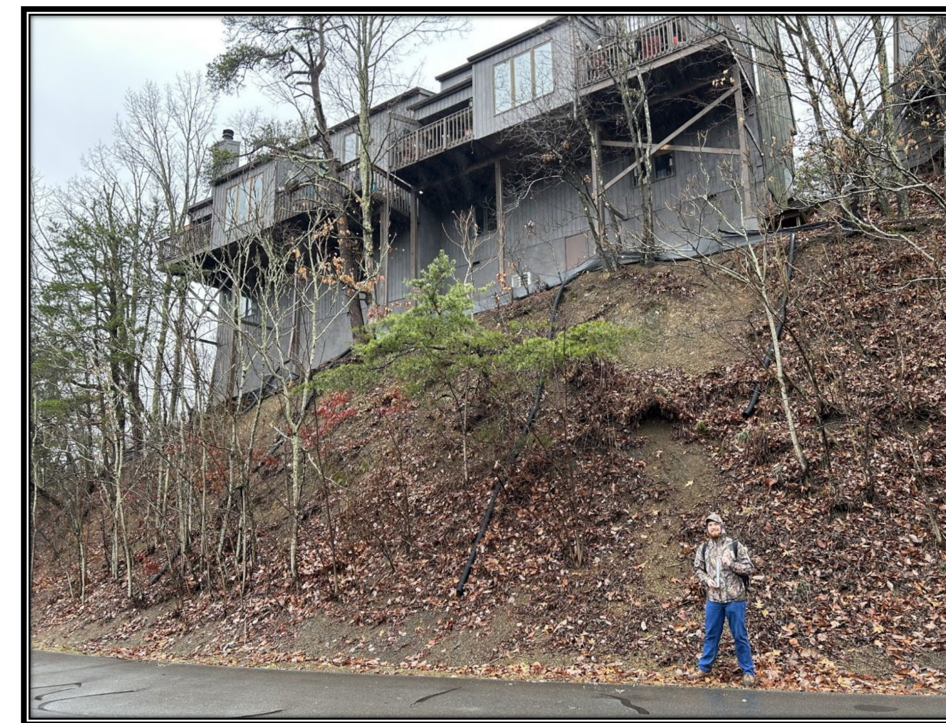
Figure 4: A picture of a steep slope behind some of the houses, the slope here was 51°.
