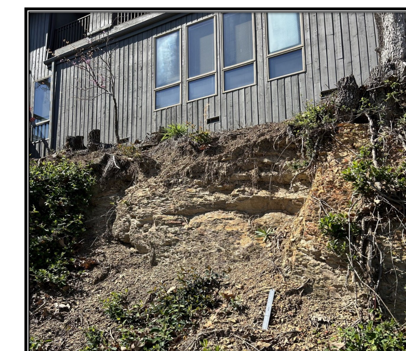
Figure 6: A steep slope showing outcrop of Sevier Shale, this area has had slope failures as recent as 2022.
