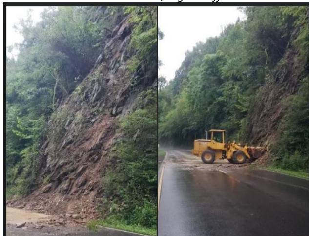
Cleanup of the rockslide on the Spur in Sevier County. Source: Facebook post from Sevier County Emergency Management Agency.
