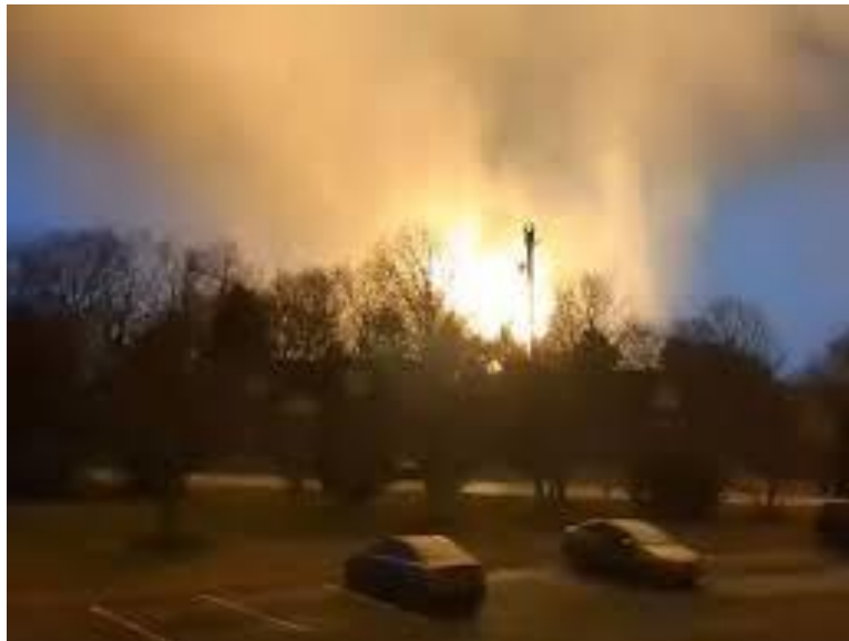
A large explosion was caused when the tornado hit an NES substation in Madison, TN. Image via: BrandonDavisBD/Twitter
