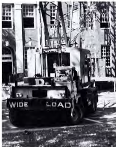
(Debbie Morton) The sign on the crane says it's a wide load, and you had better believe it!!! Roads might get blocked during the renovation.
