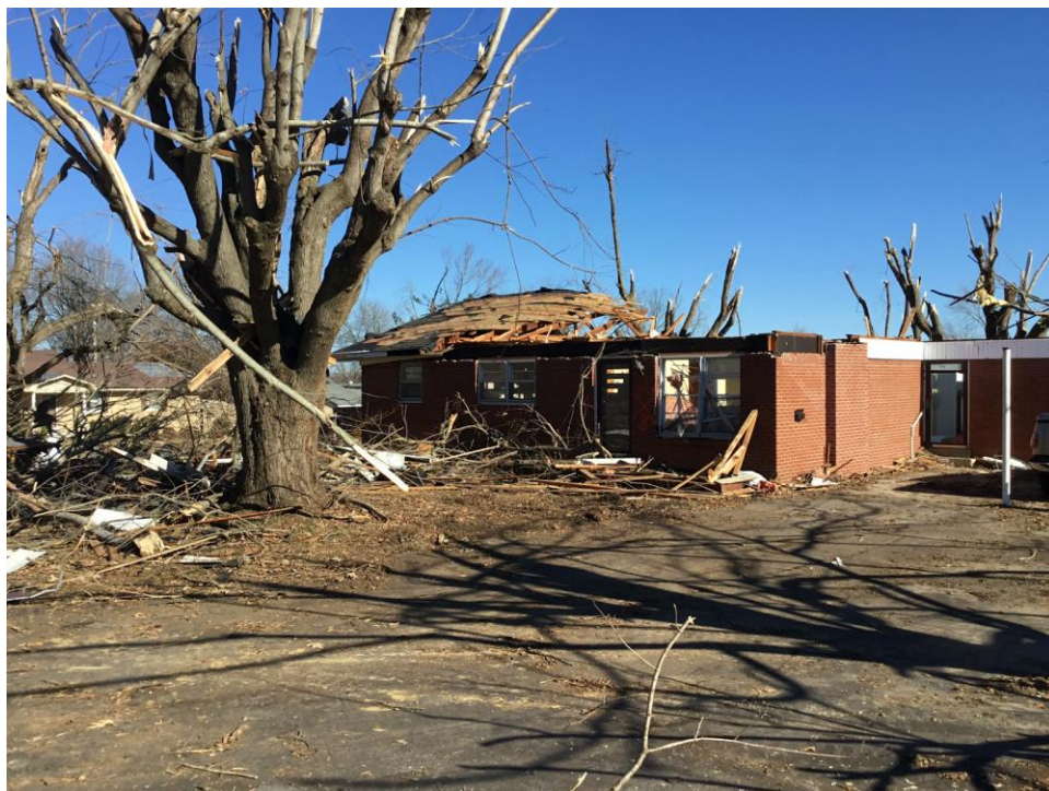
EF-2 tornado damage in Kenton, TN. (NWS-Memphis)
