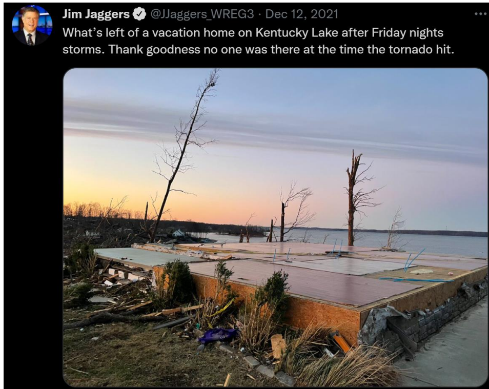
Tornado damage on Kentucky Lake (Jim Jagers, Twitter)
