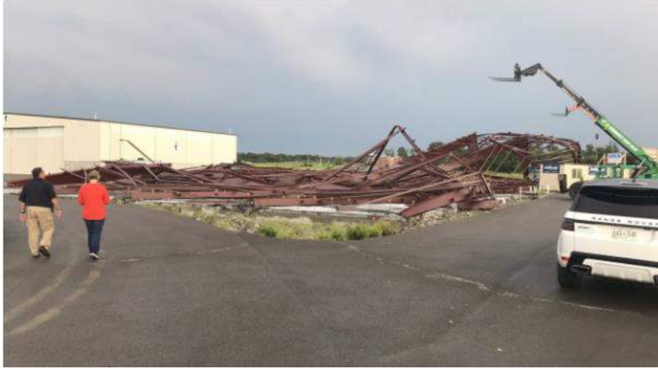
Damage to a hanger under construction at the Lebanon Municipal Airport in Wilson County. Image via News Channel 5 Nashville.
