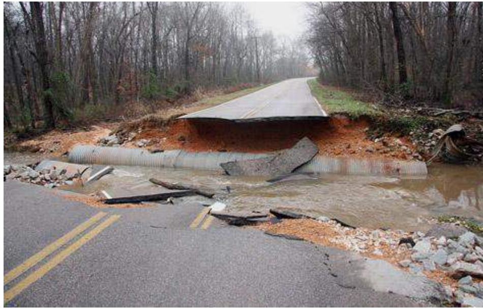
Reynoldsburg Road washed out and impassable near Paris, TN (Henry County). Photo via Ron Park, The Paris Post Intelligencer.
