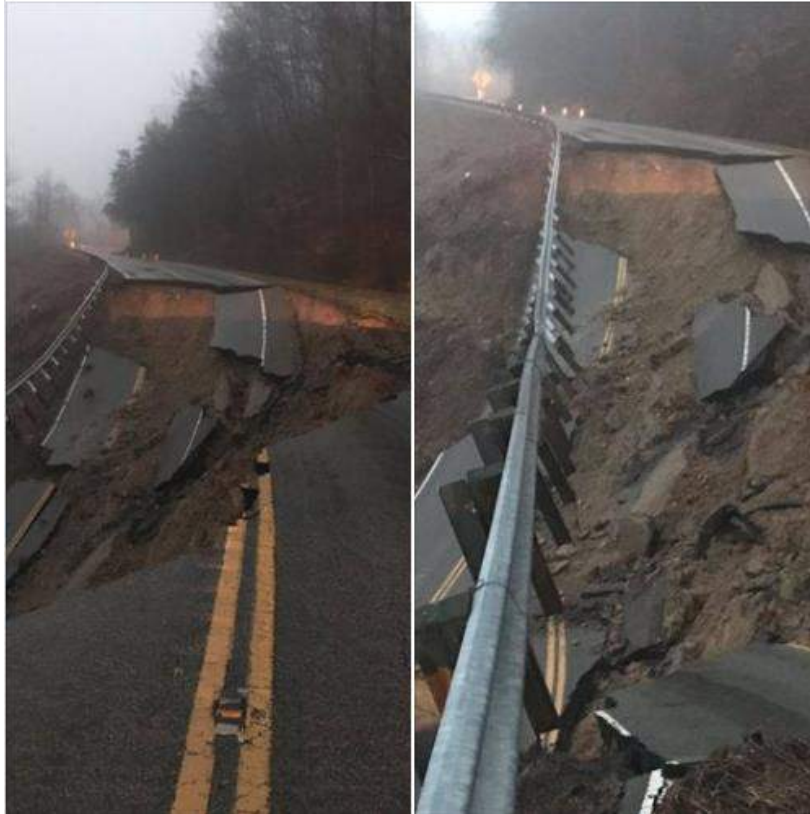
Damage to Hwy 70 in Hawkins County, due to a mudslide which occurred Feb 21 st and proved fatal. Photo via Mark Naigi (TDOT).
