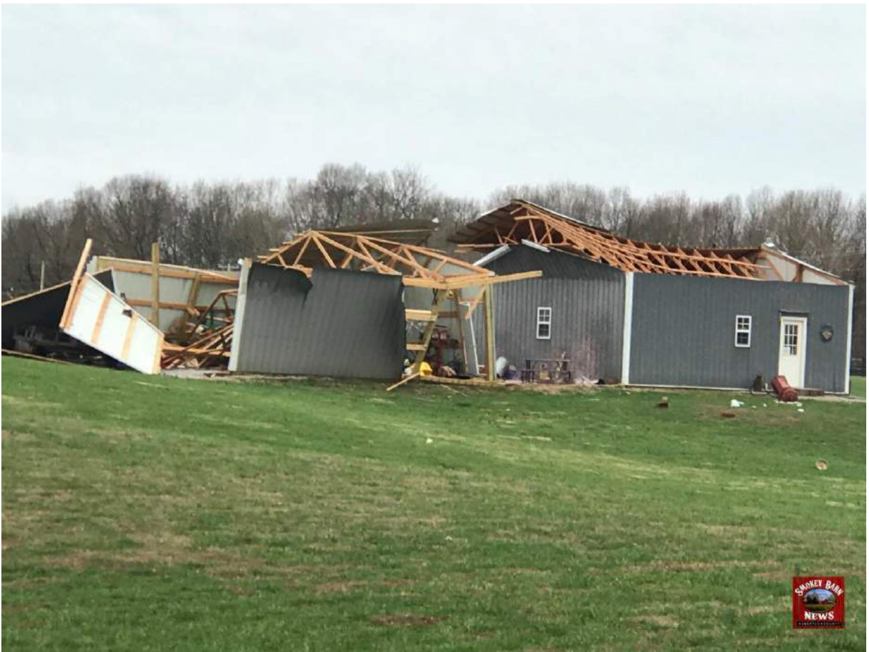
Tornado damage in Robertson County (via NWS Nashville Facebook Page)
