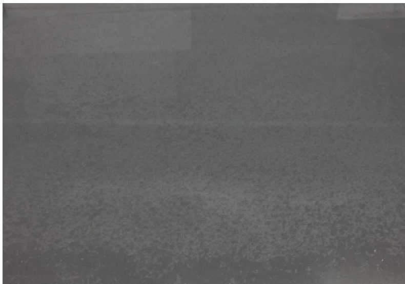
Figure 30. Entrapped Air Bubbles Resulting from Aerosol Application of Klean Strip®
